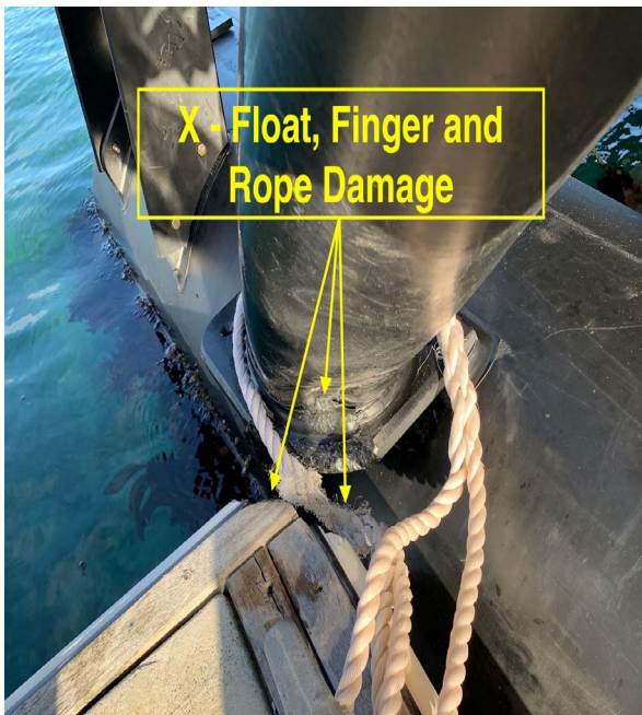
Pic I. Non-Compliant Installation. (Pontoon)
