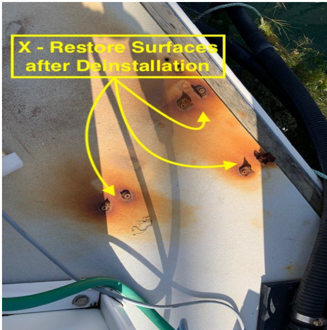
Pic M. Non-Compliant Decommissioning.
